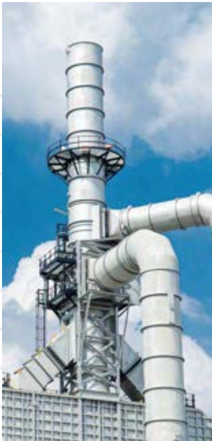
MISSION CRITICAL APPLICATION
